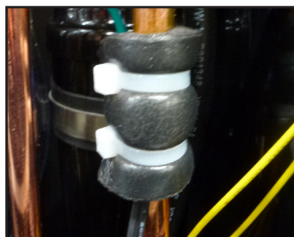
Figure 6: Thermistor attached to the refrigerant line.
